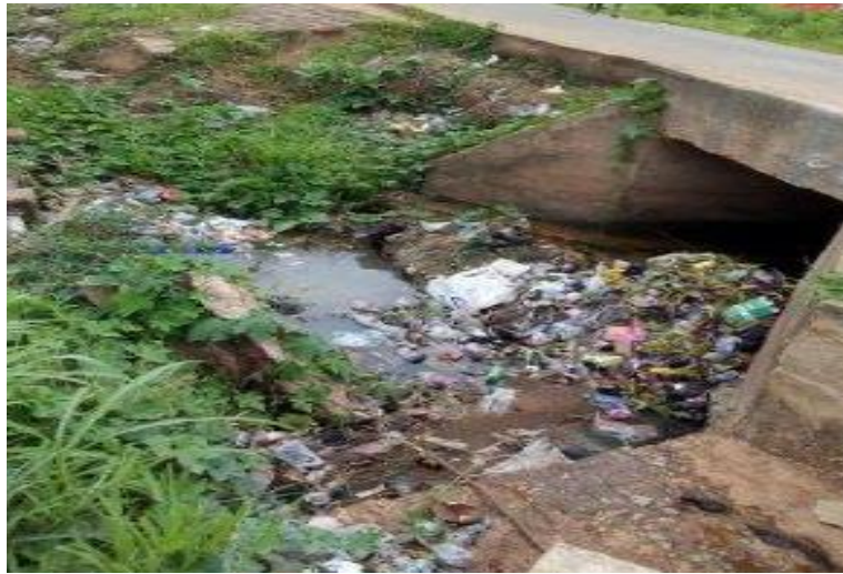
Figure 6: A Drain being choked by illegal dumping of waste
